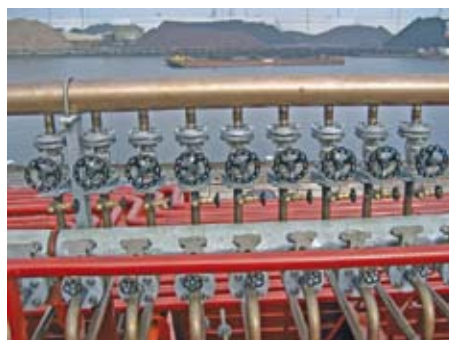
View of the new above the existing header. Also on view are the shut off valves for the individual heating coils
