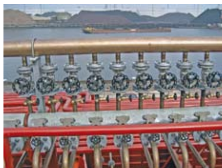
View of the new above the existing header. Also on view are the shut off valves for the individual heating coils
